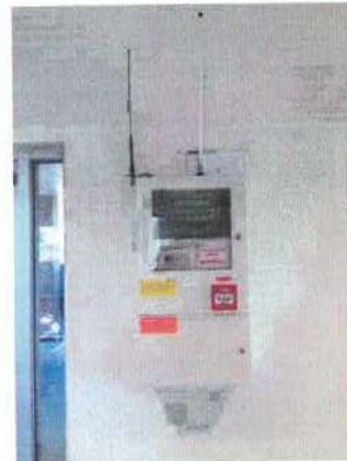
Figure 2.5 – Fire Indicator Panel
