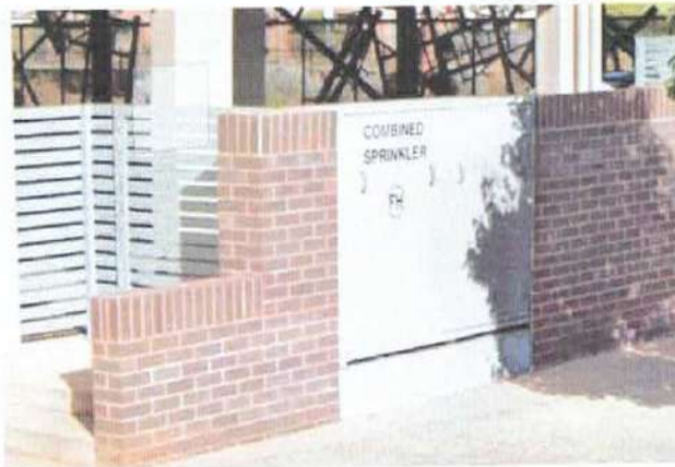
Figure 2.4 – Combined Fire Hydrant & Sprinkler Booster
